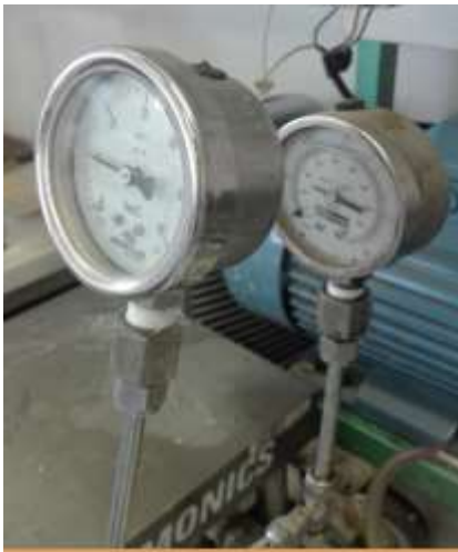
Figure 3.7 Manometers installed at the entrance and exit of the membrane module
