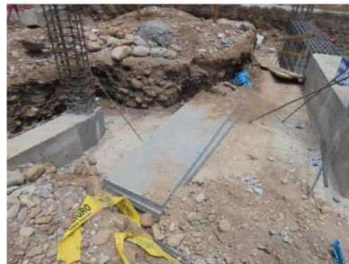
Figure 2.10. Surplus formwork partially buried on site
