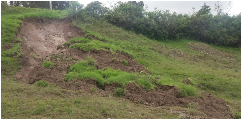
Figure 37.- Slope failure after a suddenly – heavy rain, Cajamarca, Peru/2019.
