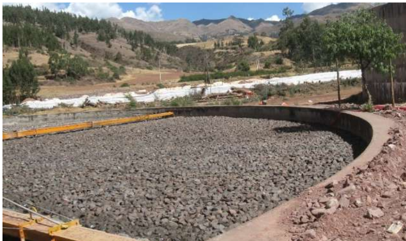
FIGURE 3.6 OLD TRICKLING FILTER (ROCK MEDIA). THE PHOTO WAS TAKEN ON 2012
